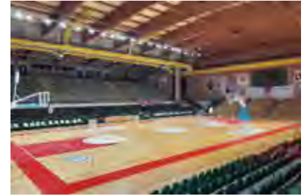
In Sep, 2021, our ENELTEC LED Stadium Lights were used in a basketball court in Italy , customer used the 30 degrees beam angle and confirm the lighting effect is perfect.
